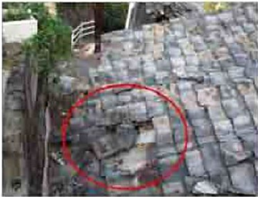
A case where some roof tiles have detached or shifted, causing water leakage.
