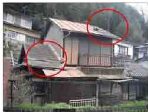
A case where part of the asphalt roof has shifted, causing water leakage.
