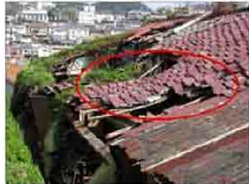
A case where the columns and beams are severely damaged or deformed, posing a risk of collapse.
