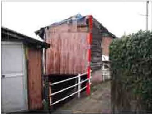
A case where some columns are tilting.
