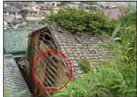
A case where the exterior wall has peeled off, severely exposing the underlying surface and creating holes that penetrate the wall structure.
