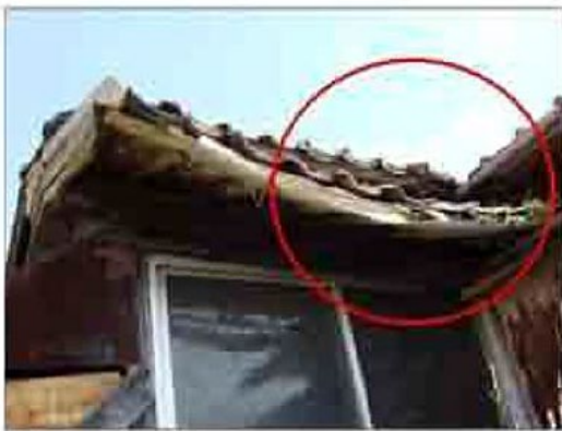
Case where part of the asphalt roof has shifted, causing water leakage.
