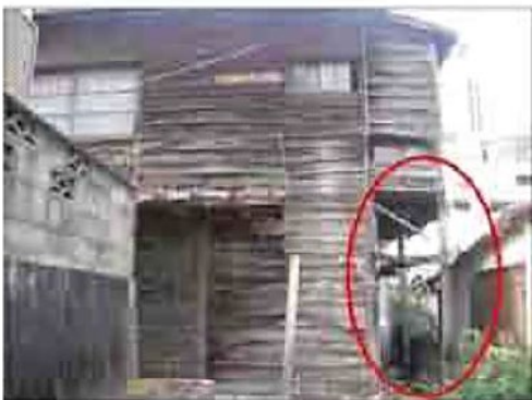
A case where multiple parts of the column are damaged.
