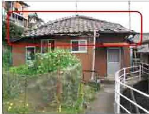
A case where the eaves' baseboard and supporting wood have deteriorated, causing the eaves to sag.
