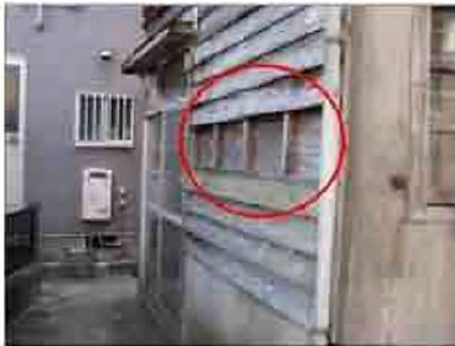
A case where part of the exterior wall finishing material has peeled off, exposing the underlying surface.
