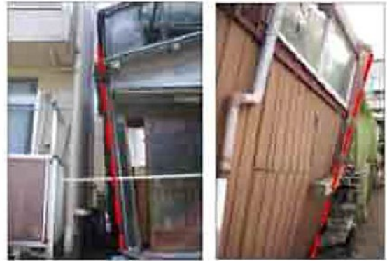
A case where column deformation is severe. There is a risk of collapse.
